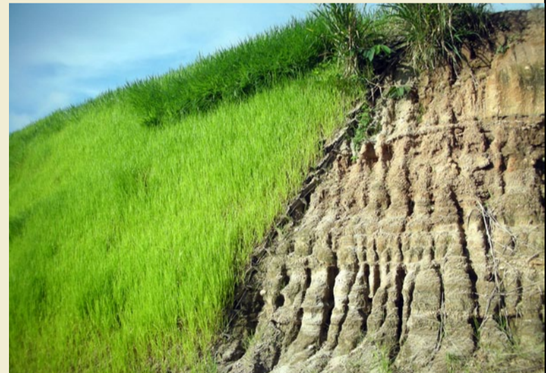
Finished Project showing termination of material (Left is complete, Right is original slope)
