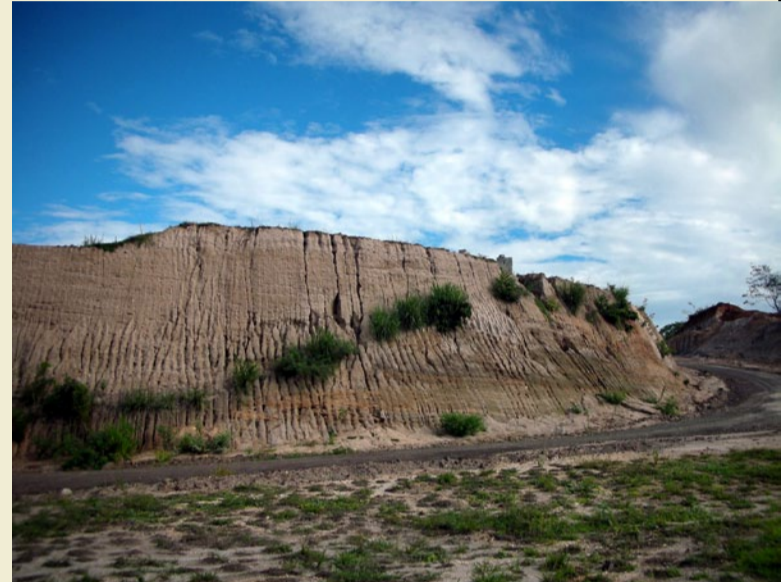
Punta Raton Beach Properties (Pre-Envirogrid Slope Erosion Control System)
